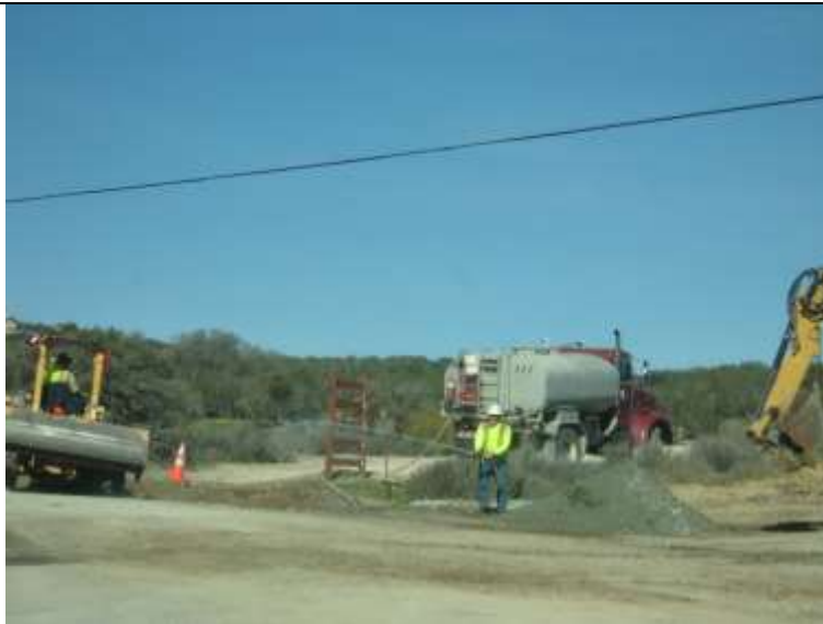
Photo 2: In accordance with MM-BIO-4a and MM-AQ-1, crews were active in spraying down curb grade work along the underground alignment with water to minimize dust emissions.
