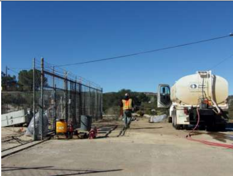
Photo 4: Fire tools and fire watch were on site during existing Boulevard Substation Demolition as stipulated by MM-FF-1.
