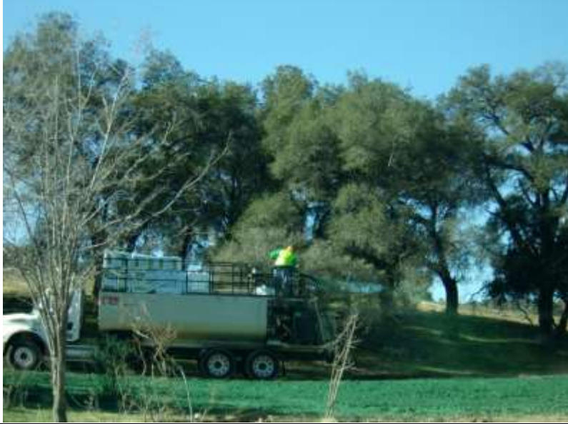
Photo 3: Temporary work areas within Boulevard Substation were restored and hydro-seeded in accordance with MM-BIO-1d and the Habitat Restoration Plan.
